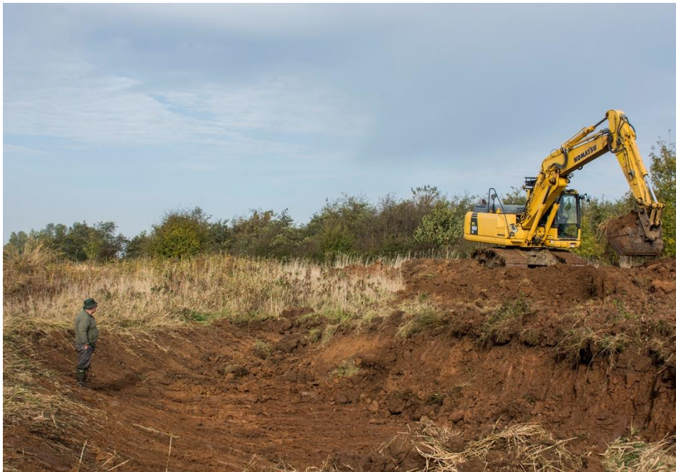
Peter Cook supervises work on a new pond at Hollym Carrs Nature Reserve. Autumn 2016 – Peter Martin
